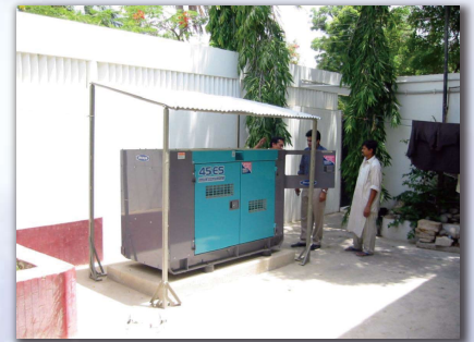
As the Emergency power source in the hospital.
